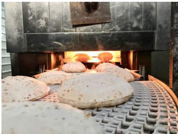
Jubata Bakery The bakery produced approximately 15,000 loaves of pita per day, serving a population of over 40,000 people. MFA shipped all of the bakery equipment from Turkey.
